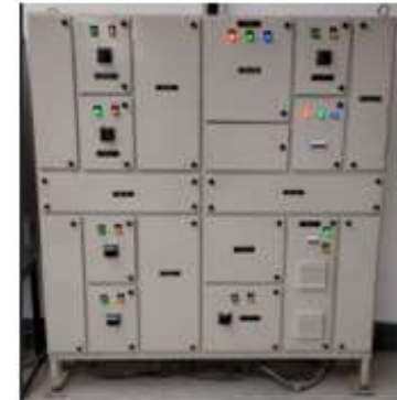
MCC PANEL +DRIVE
